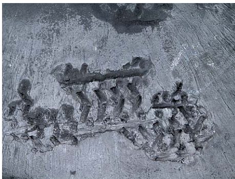
Spalled coating showing localized, sub-surface inter-bundle porosity.
